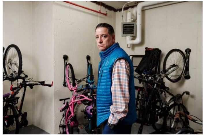
Sam LaMontanaro , director of engineering for Aufgang Architects , in a bike room in Hell's Kitchen. "A bike room is at the lowest part of the building and has the greatest water pressure for a sprinkler system," he said. Karsten Moran for The New York Times
